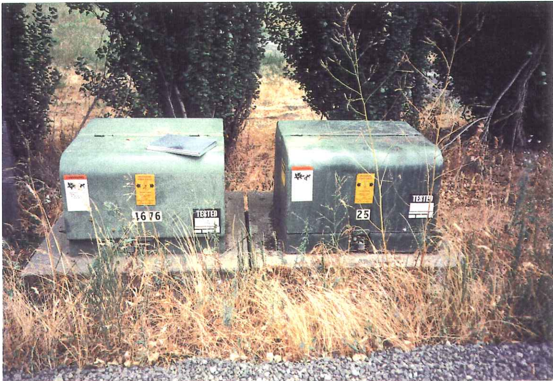
Pad-mounted Transformers (#2 and #3)
