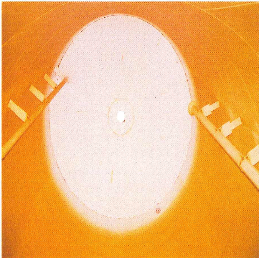
Figure 6. Corrosion staining of roof plate lap joints was observed at the interior of the tank.
