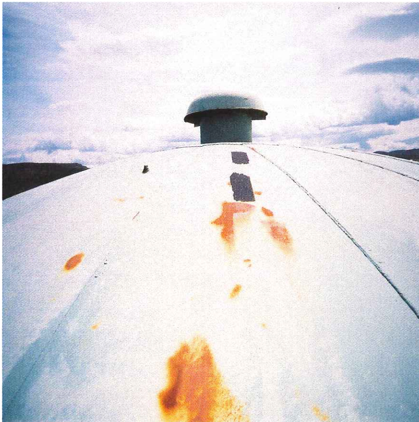
Figure 8. Thinned and worn exterior coatings were most severe at areas of the exterior roof plate.
